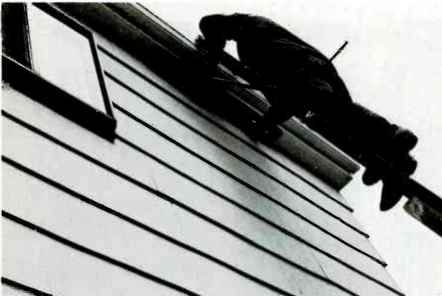
Fig. 7 Secure the 2X4 to the house, using the nails and lag screws.
