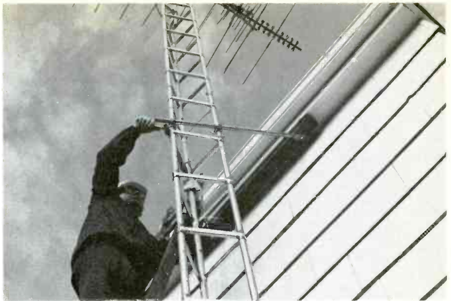
Fig. 9 A tower bracket was fastened to the tower using "U" bolts, and to the 2X4. Now, the tower was reasonably secure, but not perfectly vertical.
