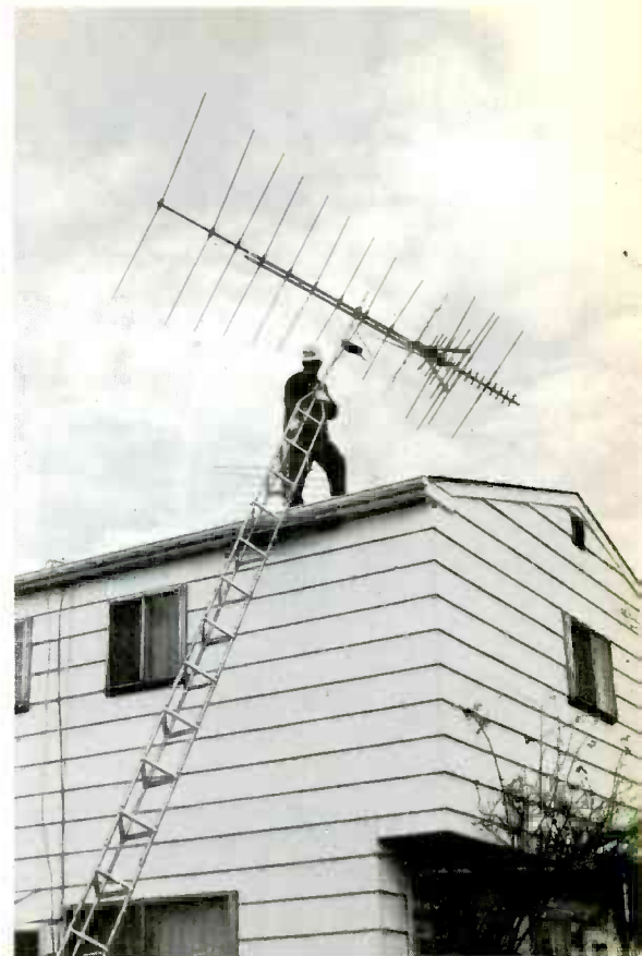
Fig. 8 The man on the roof lifted the assembled mast and antenna, connected a safety rope to prevent it from falling accidentally, and both men positioned the tower approximately where it should go.
